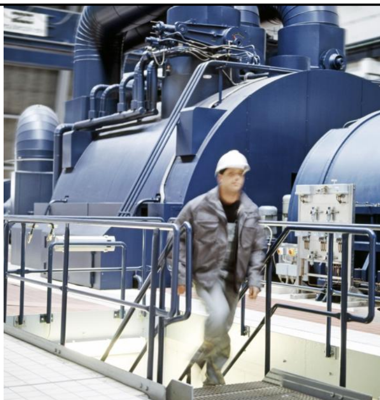
The lone worker can now rest assured that he is protected through his TETRA hand set. It also helps him in his daily work with handling technical alarms.
